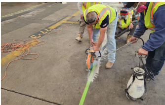
Clean cuts are made around the perimeter of area to be repaired.
