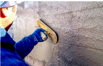
A standard pool trowel, is used to spread the Surface Armor™ and achieve an even thickness.
