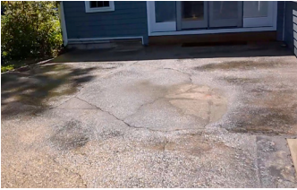
Damaged and unsightly concrete patio prior to resurfacing.
