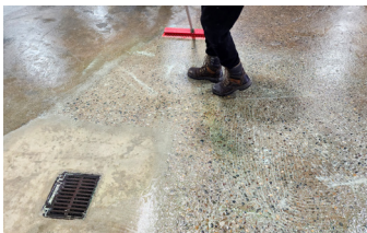
Constant vehicular traffic in a refrigerated wet environment has caused extensive wear.
