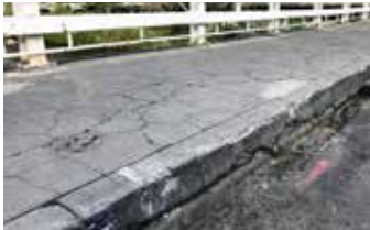
Badly cracked and spalled concrete sidewalk.
