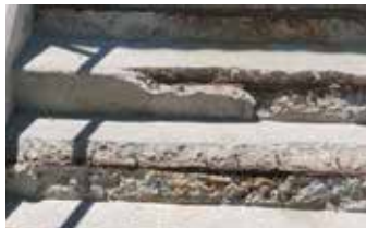
Concrete stairs degraded down to exposed steel.
