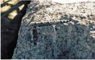
Spalled concrete with exposed rebar.
