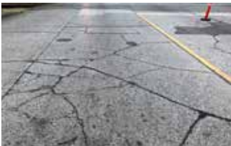
Distressed concrete roadway.
