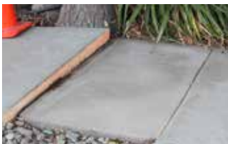
Extreme trip and fall hazard.
