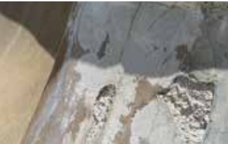
Damaged concrete surface unsafe for use.
