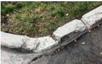
Severely damaged curb.
