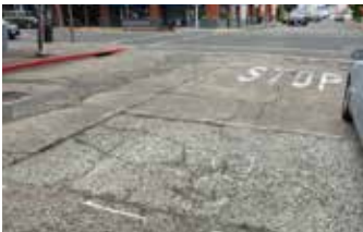
Failing road panel.
