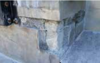
Extreme damage to loading dock.
