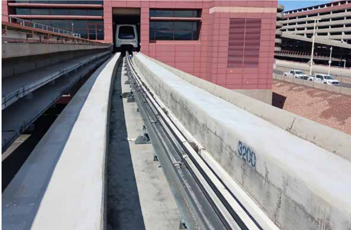
Surface Armor™ replaces traditional epoxies for long lasting, visually attractive appearance and functions at a reduced cost and expedited timeframe.
