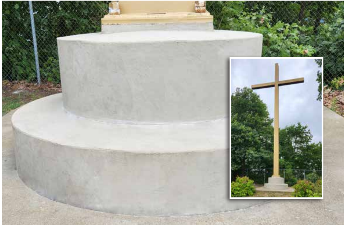
Surface Armor's ease of use and quick set time, allowed the base to be permanently repaired with a minimum disruption to the sanctuary in less than 2 hours!
