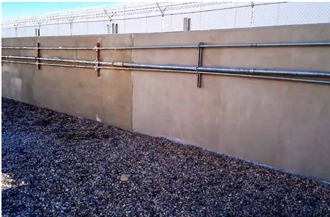
A newly resurfaced CMU block wall with a 'like new' appearance, eliminating the visual cracks and discoloration. The wall is now waterproof and structurally sound.
