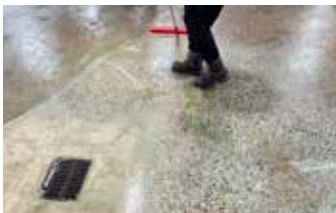
Constant vehicular traffic in a refrigerated wet environment has caused extensive wear.
