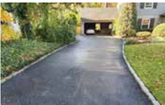
Worn out asphalt driveway prior to applying Surface Armor™.
